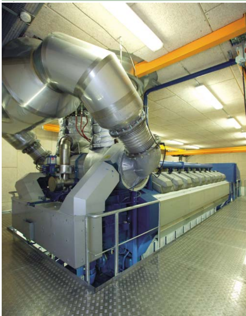
Ringkøbing Fjernvarmeværk in Denmark is powered by a Wärtsilä 20V34SG engine.
