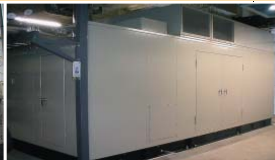
Fig. 3 Energy service in a hospital.
