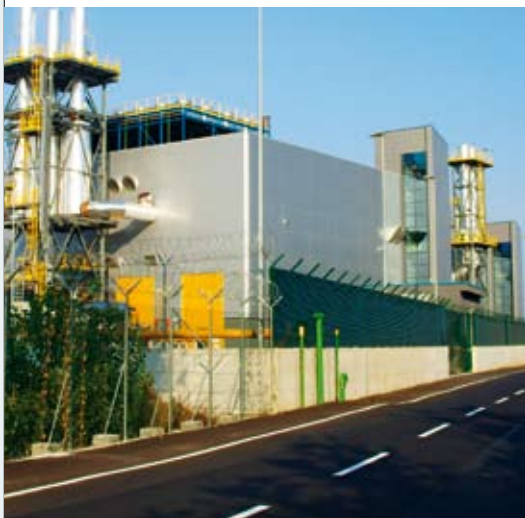
Hot water produced by the Linate CHP plant is used for district heating and to provide cooling in air-conditioning systems.
